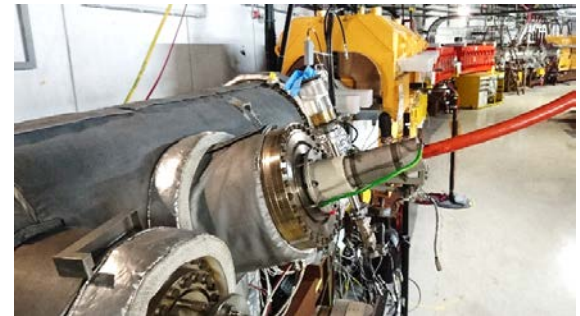
High voltage feedthrough
