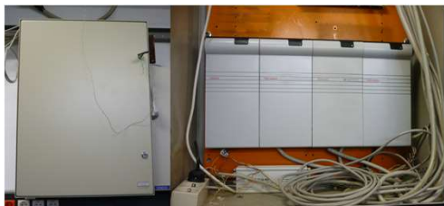
Pager System Cabinet
