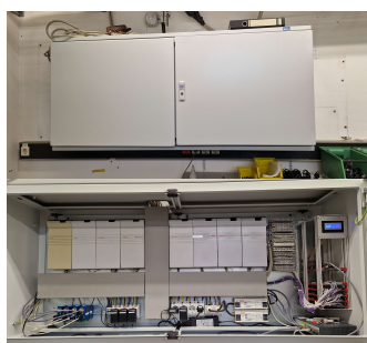
Pager System Cabinet with Connector Box
