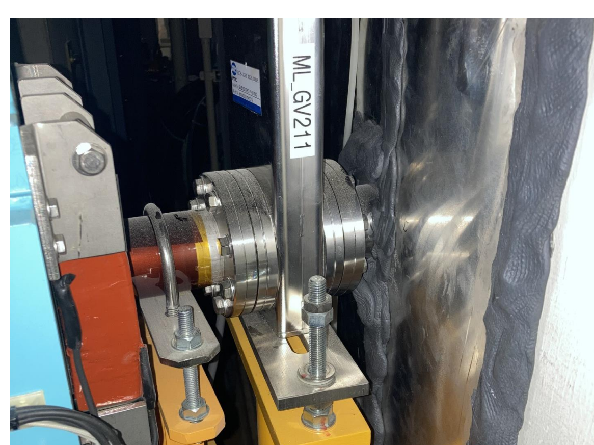
The duct that have been misaligned by the magnitude 9.0 earthquake in 2011 (according to old-timer)
