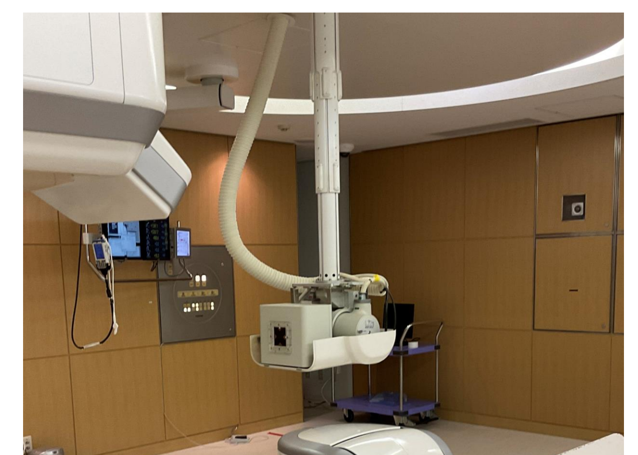
The X-ray tube suspended from the ceiling
