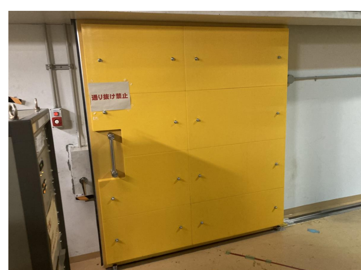
The door that open a few centimeters every time when an earthquake occurs
