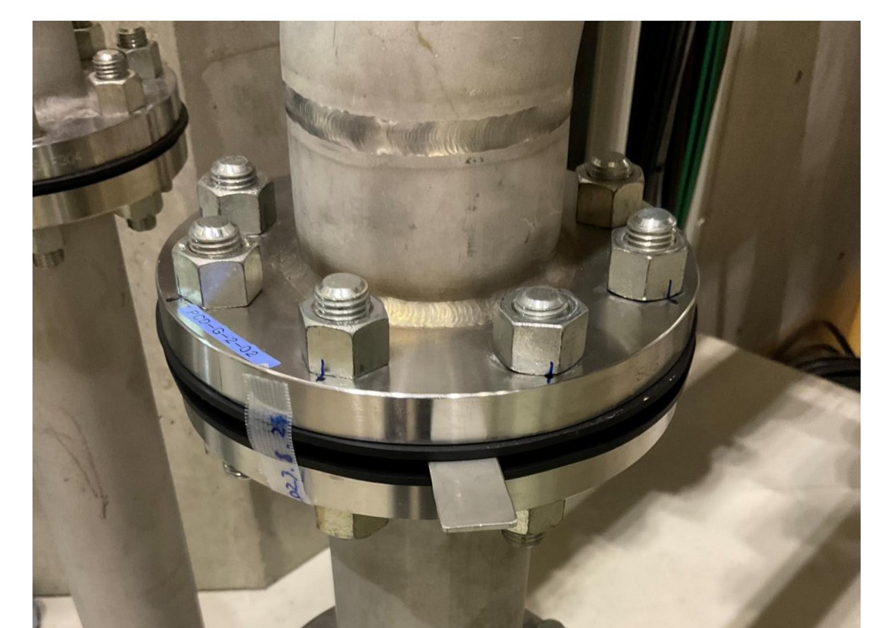
The flanges sealing coolant piping
