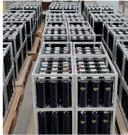
Capacitors for energy recovery
