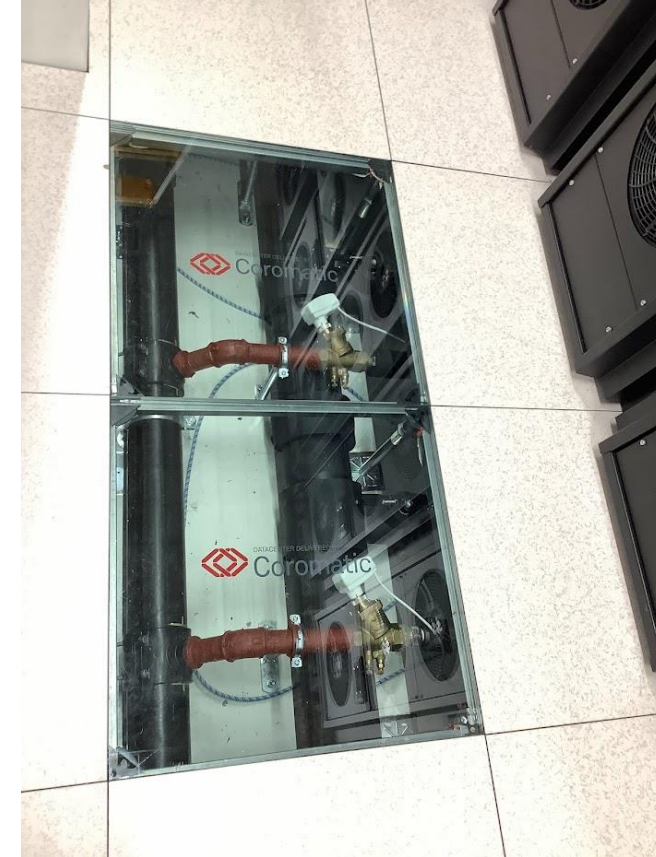
Efficient cooling within racks by a large scale water cooling system
