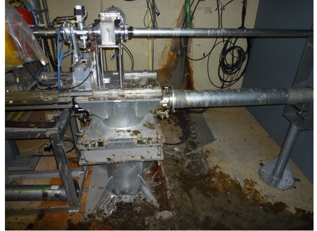
Figure 4: Damage to the injector linac tunnel caused by the earthquake. Quadrupole magnets fell from its support stand ( upper ), and groundwater gushed out at an expansion joint ( lower ). A pond is located adjacent to the west side of the injector linac, serving as the source of the groundwater.
