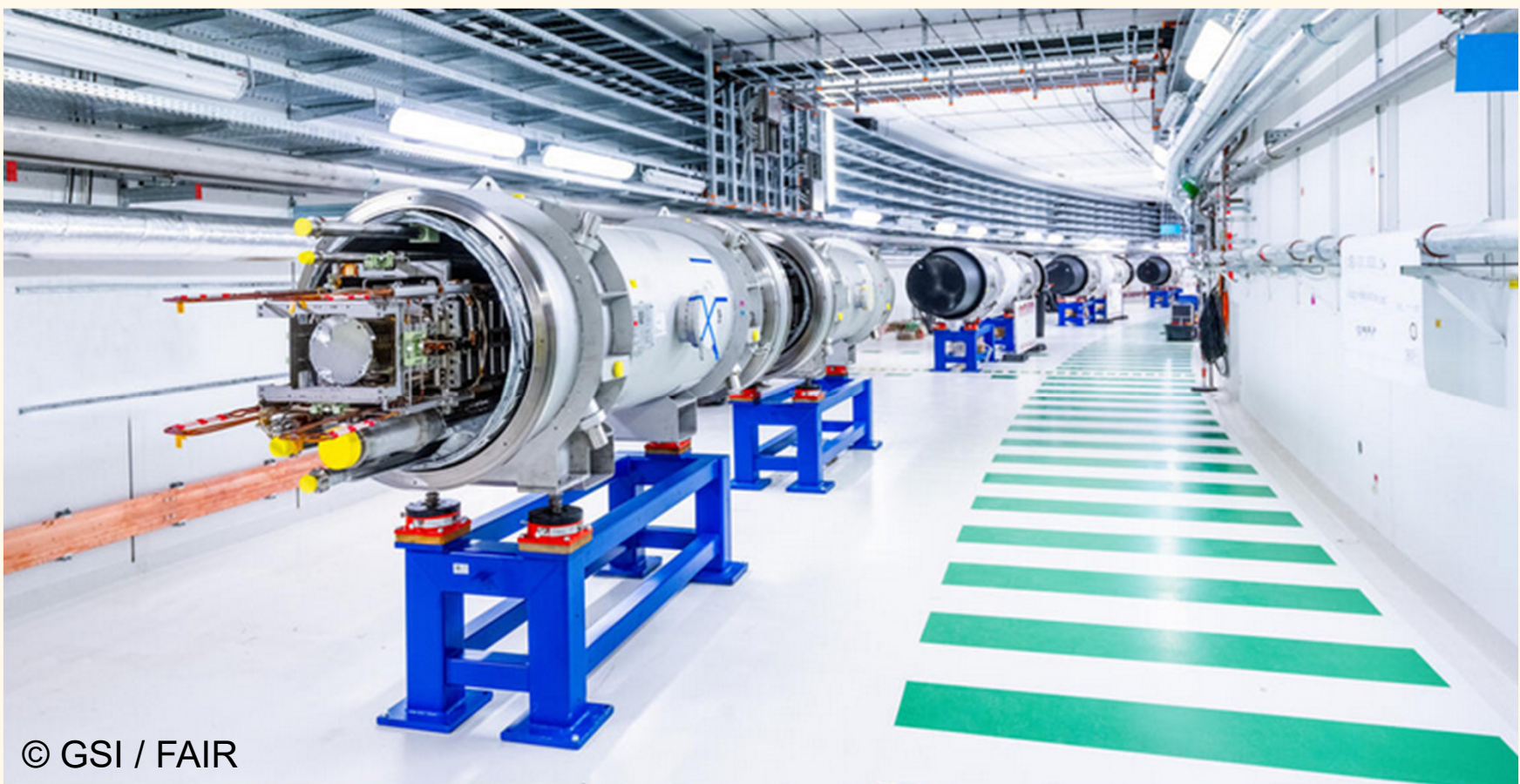
SIS100 curve section – installed superconducting dipoles (CDM) on the blue-line
