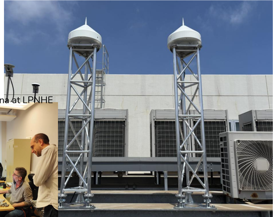
GNSS Antenna installed at JPARC Neutrino building
