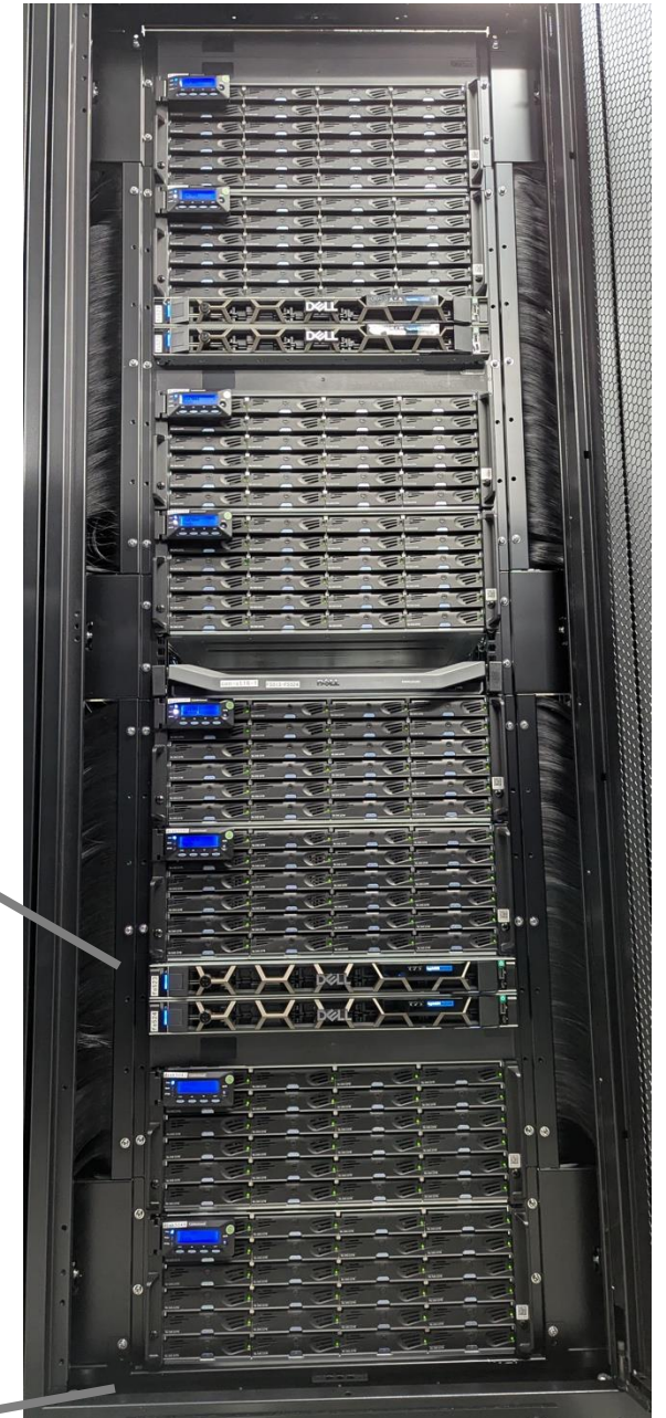
Storage Server Rack
